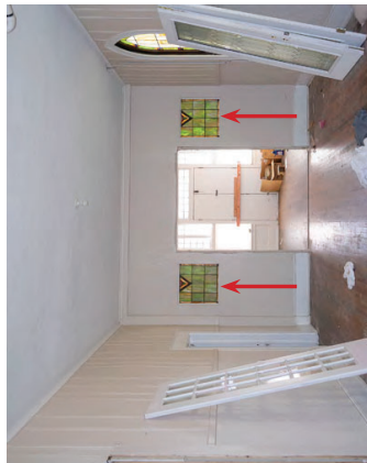
The two surviving sashes (red arrows) were installed in the nonhistoric demising wall outside of the Period of Significance according to Evelyn Kennebrew, who lived above the funeral home with her parents in the mid-century.
