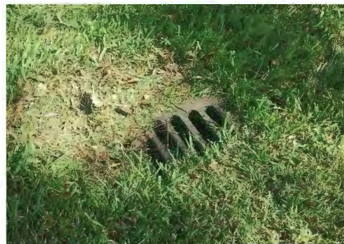
Figure 6 Clogged Inlet Grate
