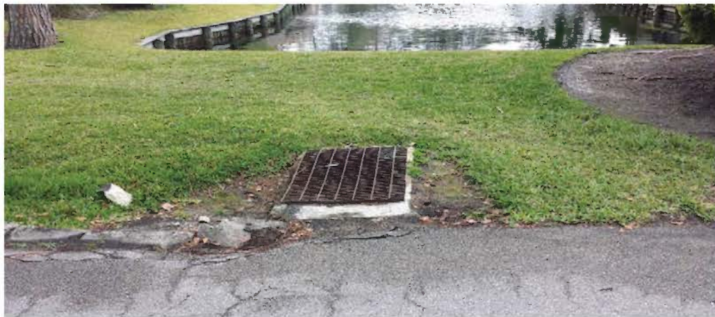
Figure 3.2 Failing Drainage Structure and Bioswale Opportunity
