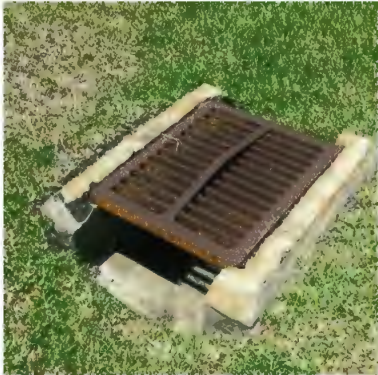
Figure 1 Failing Stormwater Infrastructure
