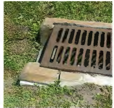
Figure 3 Failing Stormwater Infrastructure
