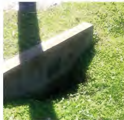
Figure 7 Clogged Driveway Culvert
