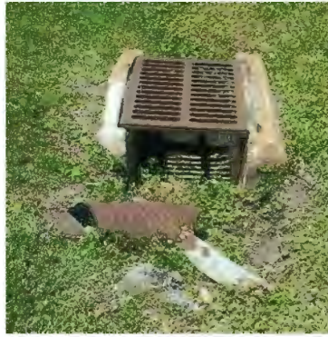
Figure 2 Failing Stormwater Infrastructure
