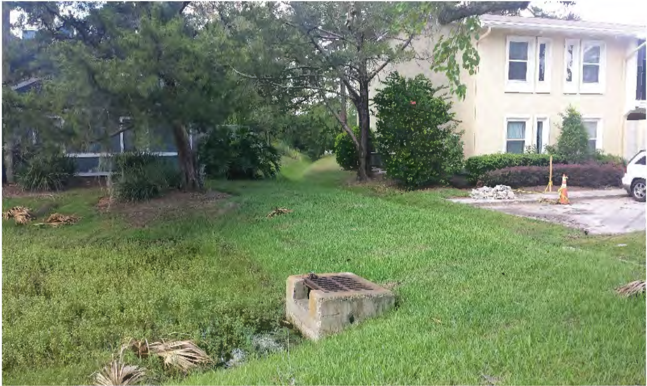
Figure 3.4 Existing Dry Retention (Left) Discharging to a Swale (Background) Draining to Lake 4
