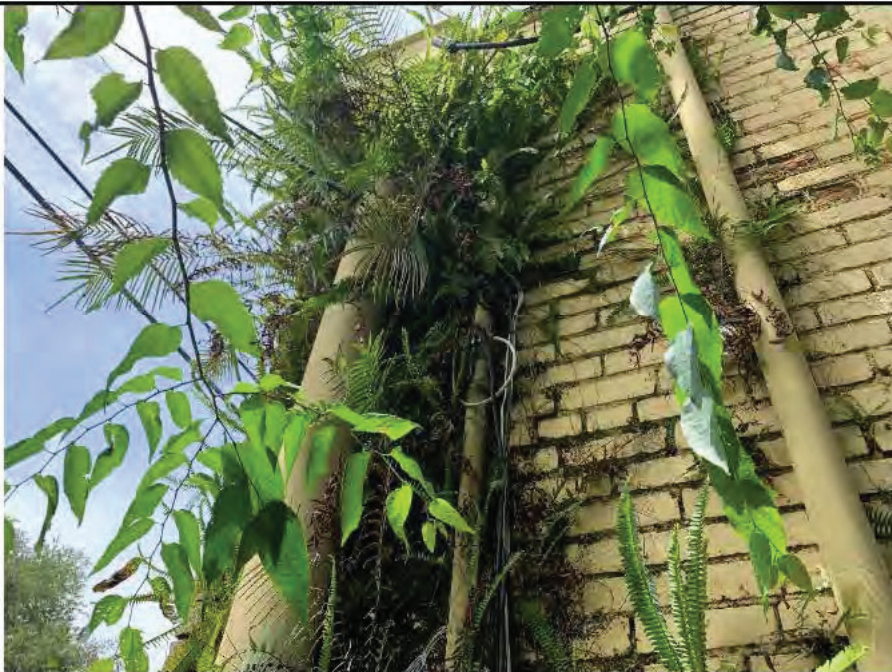
Photo 8: Heavy vegetation on southwest corner of the building. This corner has water intrusion likely from mortar damage.
