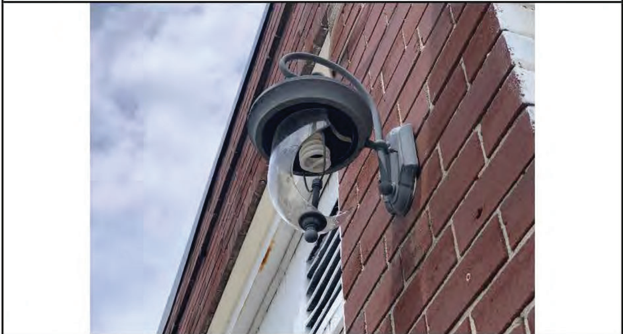
Photo 10: Broke globe at light fixture.
