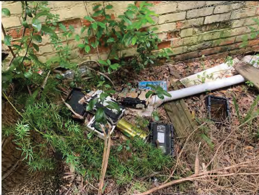
Photo 6: Damaged/missing brick masonry along south elevation.
