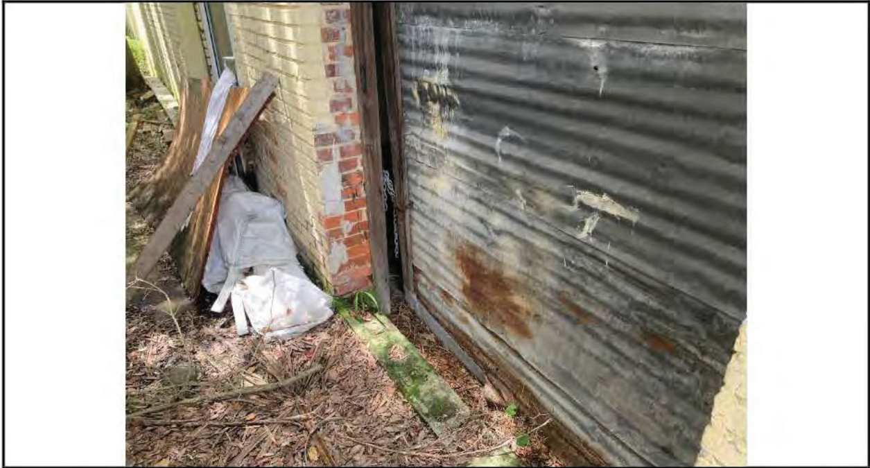
Photo 9: Southeast entry doorway which the sill is lower than the surrounding sidewalk allowing for direct water entry into the building.
