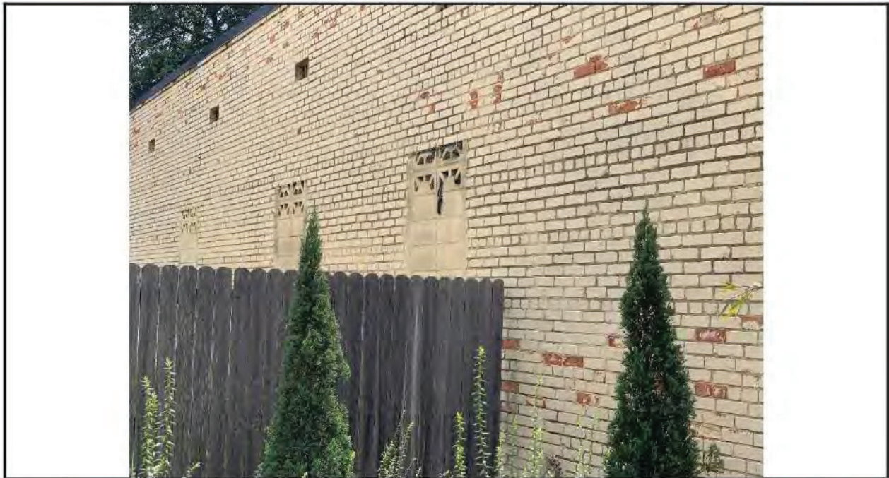
Photo 3: Partial eastern elevation – similar across entire elevation. Located along property line possibly.
