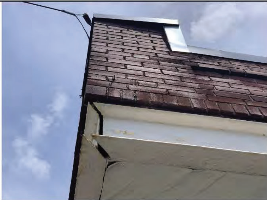
Photo 12: Northwest corner steel lintel with a gap in the connection over entry doorway.
