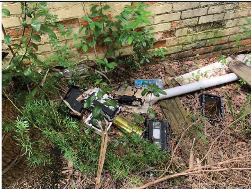
Photo 6: Damaged/missing brick masonry along south elevation.
