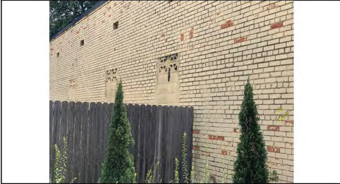
Photo 3: Partial eastern elevation – similar across entire elevation. Located along property line possibly.
