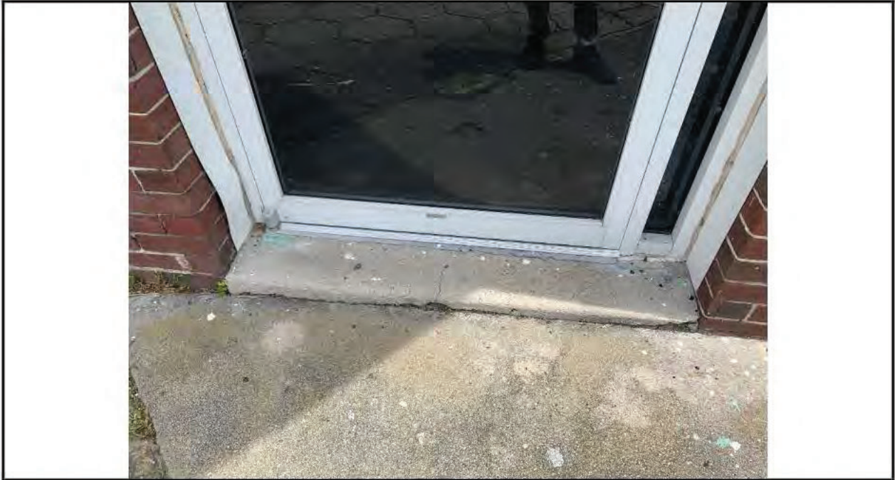
Photo 13: Typical thresholds with steps which do not meet ADA access requirements.
