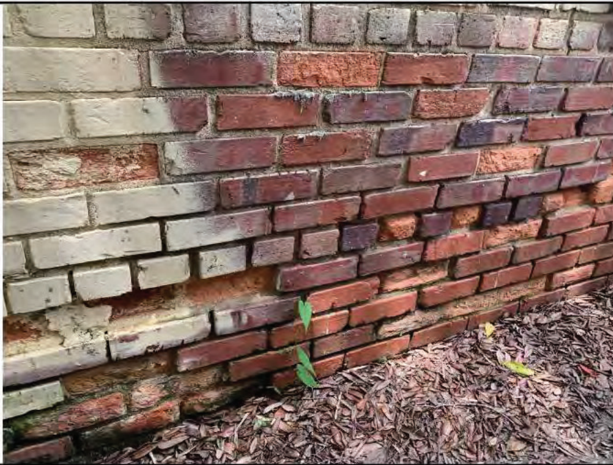
Photo 7: Damaged/missing brick masonry along south elevation.
