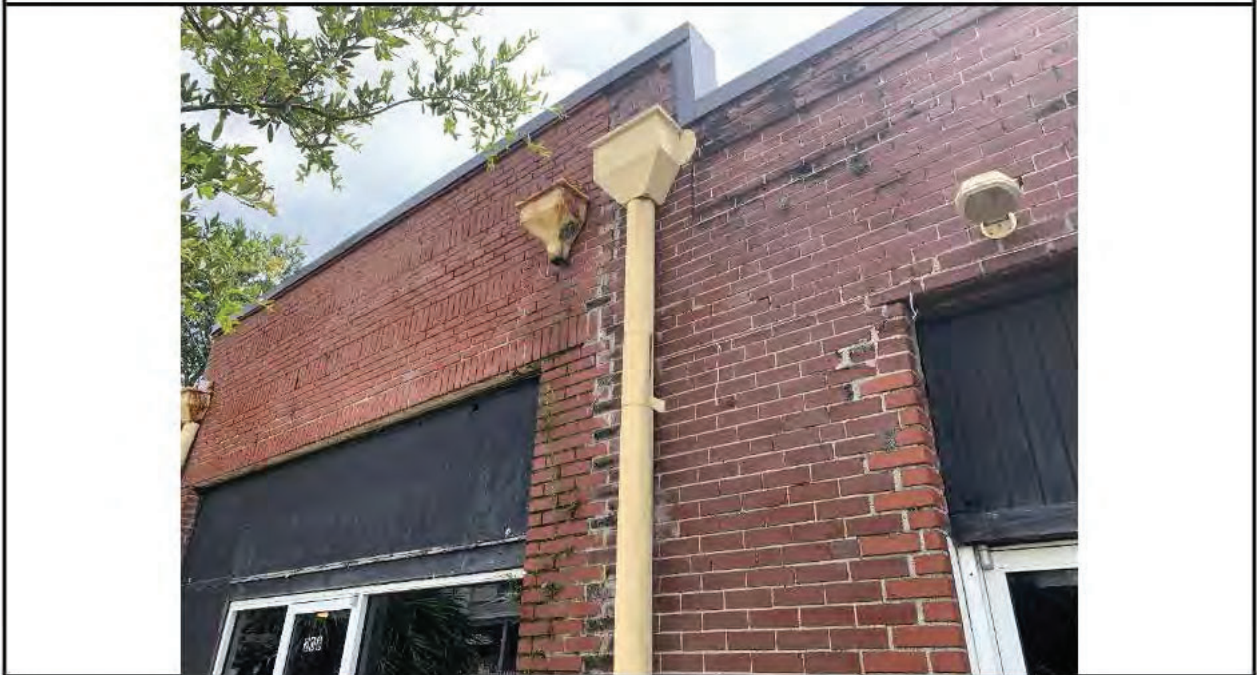
Photo 14: Current downspouts. Note poor brick mortar and heavy dirt.
