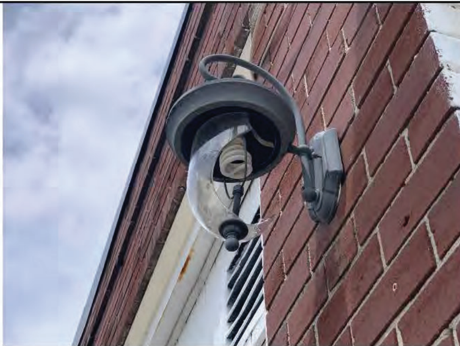
Photo 10: Broke globe at light fixture.
