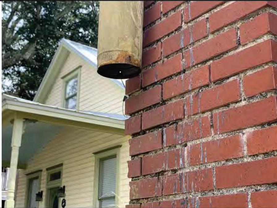
Photo 11: Section of missing downspout and mortar which is missing.
