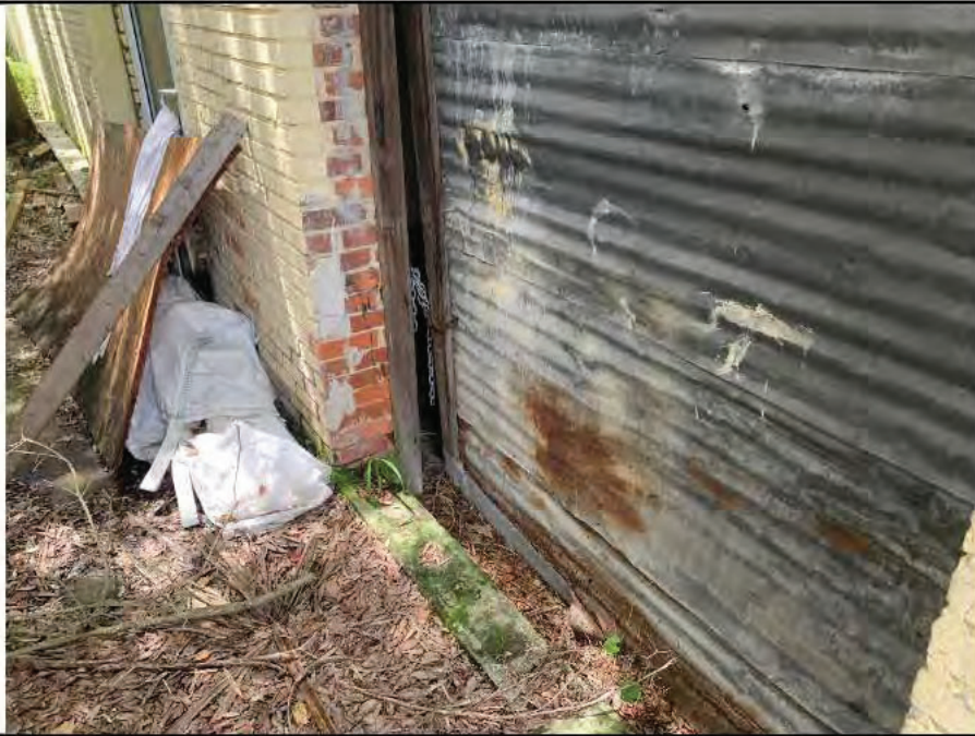
Photo 9: Southeast entry doorway which the sill is lower than the surrounding sidewalk allowing for direct water entry into the building.
