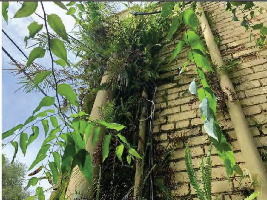
Photo 8: Heavy vegetation on southwest corner of the building. This corner has water intrusion likely from mortar damage.
