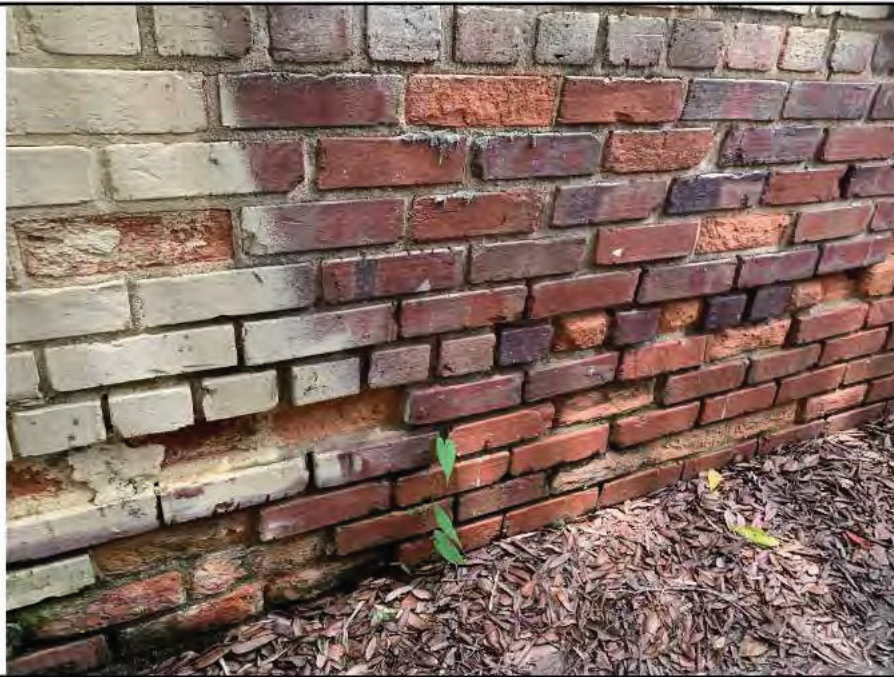
Photo 7: Damaged/missing brick masonry along south elevation.
