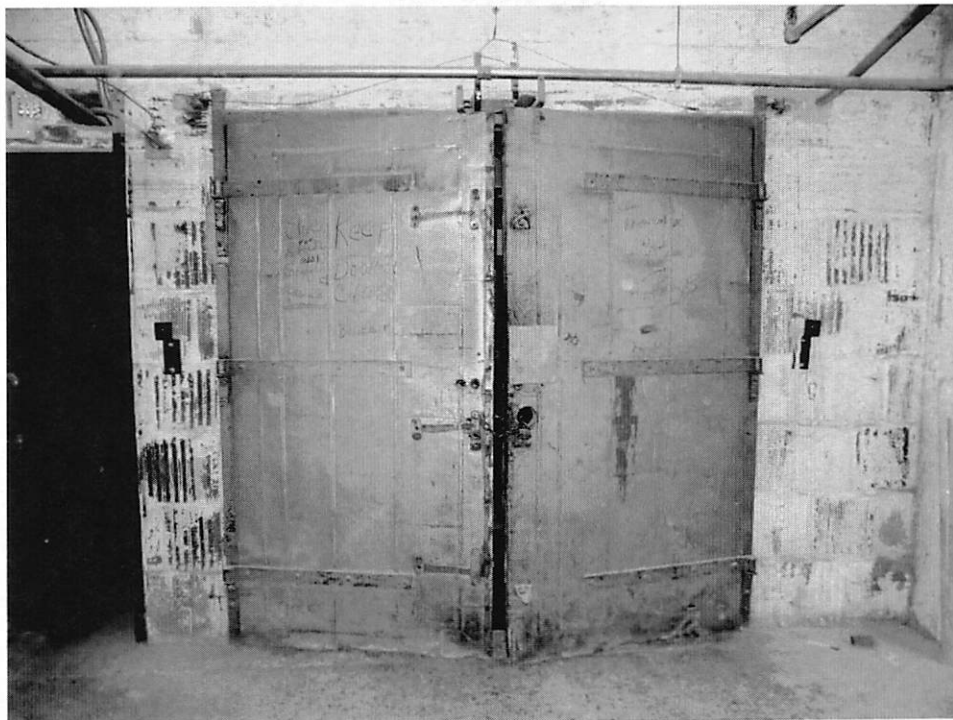
Photo 28 - Interior, basement Unit E, elevator fire shutter door, looking east.
