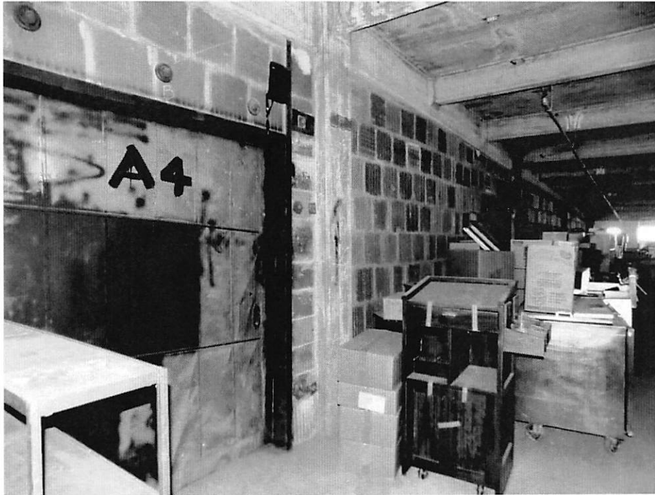
Photo 27 - Interior, fourth floor Unit A, terra cotta wall and automatic fire door, looking west.
