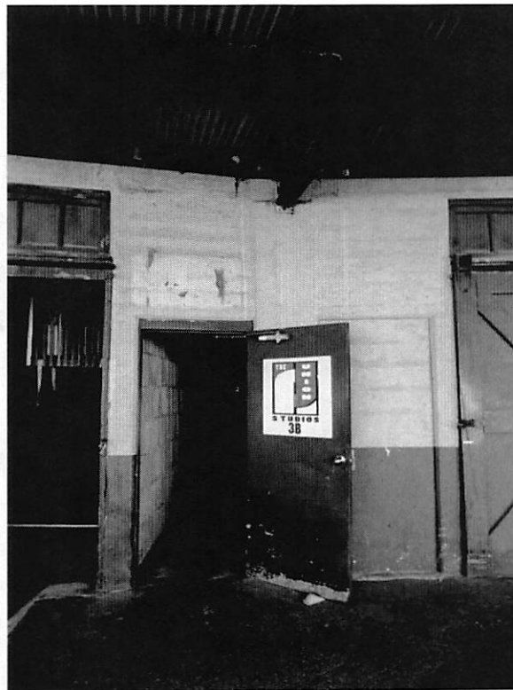
Photo 16 - Exterior, west façade (front), door into stairwell for Unit B, looking east.
