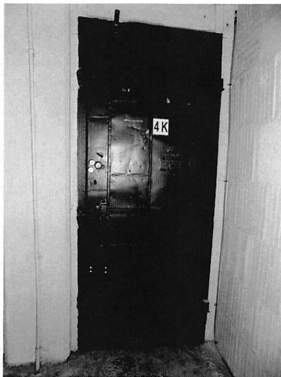
Photo 30 - Interior, fourth floor Unit K, fire shutter door from stairwell, looking east.
