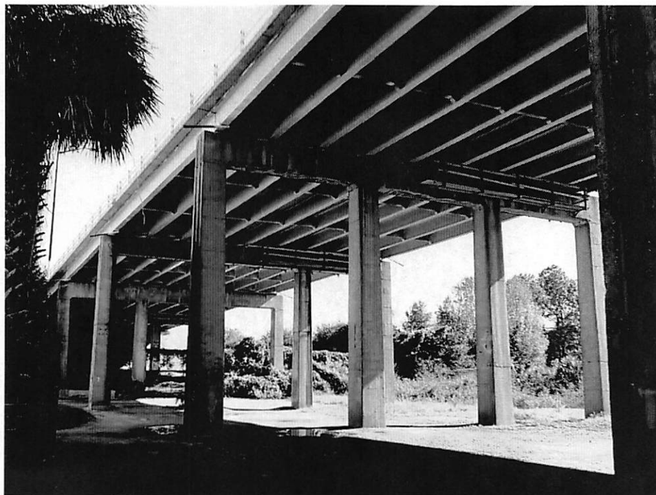
Photo 38 - Exterior, view of Arlington Expressway looking southeast from southwest corner of building.
