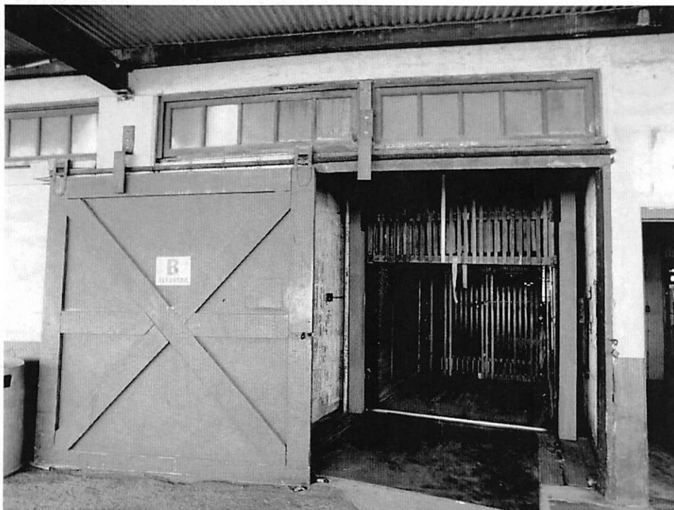
Photo 14 - Exterior, west façade (front), loading door and elevator on first floor, Unit B, looking east.
