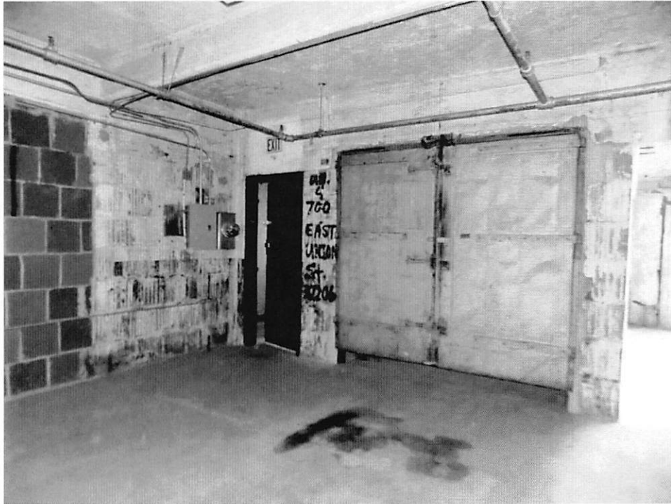
Photo 23 - Interior, fourth floor Unit E, elevator and fire shutter doors, looking northeast.
