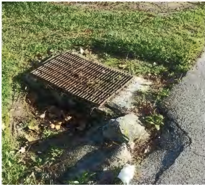
Figure 4 Failing Stormwater Infrastructure
