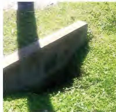
Figure 7 Clogged Driveway Culvert
