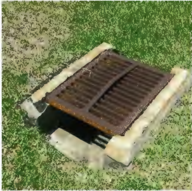
Figure 1 Failing Stormwater Infrastructure
