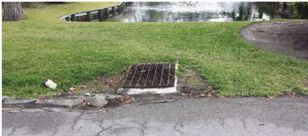
Figure 3.2 Failing Drainage Structure and Bioswale Opportunity
