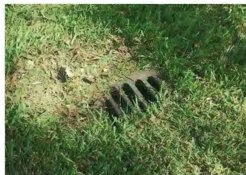
Figure 6 Clogged Inlet Grate
