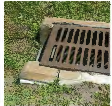
Figure 3 Failing Stormwater Infrastructure
