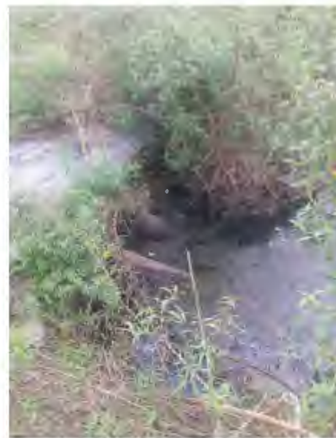
Figure 4 Clogged Lake Outlet
