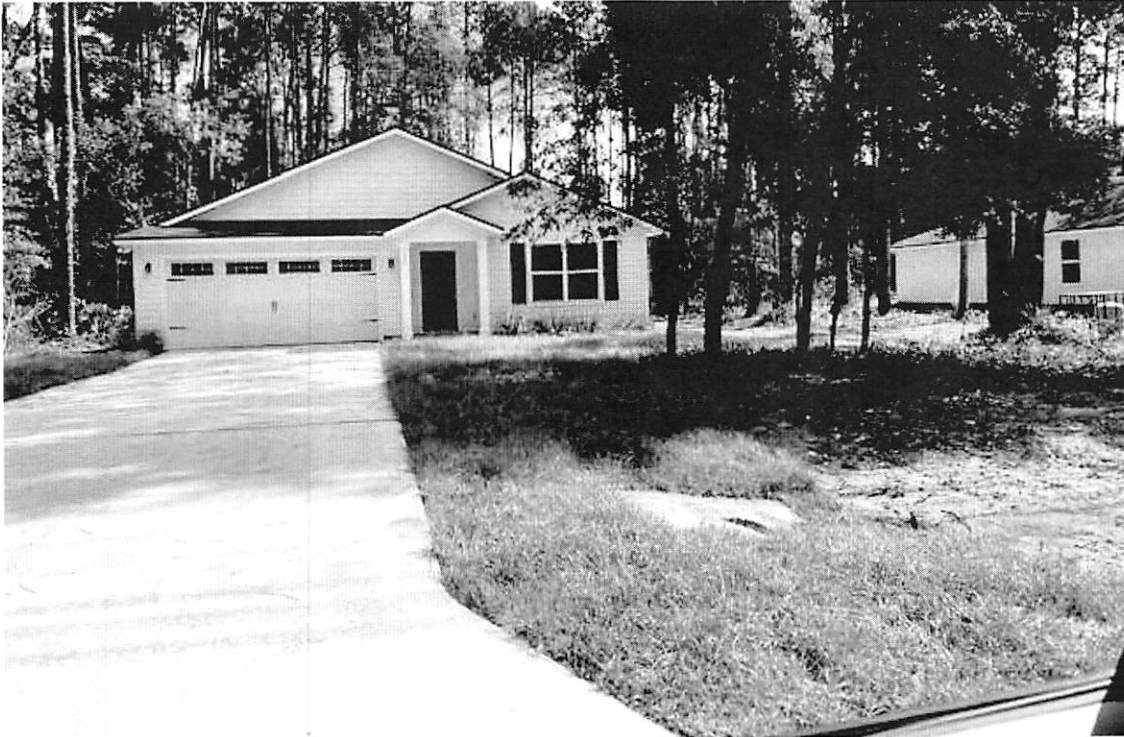
New construction of single family dwelling on Dunn Creek Road across from entrance
