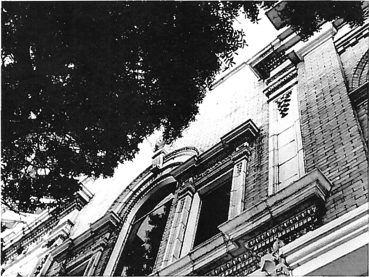
Photo 9-The W. Bay Street Parapet (due to the tree a direct shot of it is impossible)
