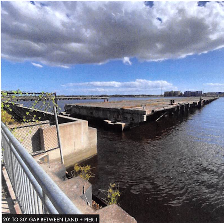
ACCESS ISSUES TO PIER 1
