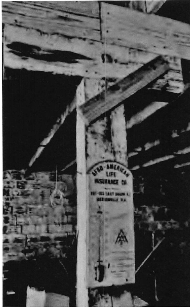
Figure 18: 2019 photograph of second floor casket factory support post, by Tim Gilmore.
