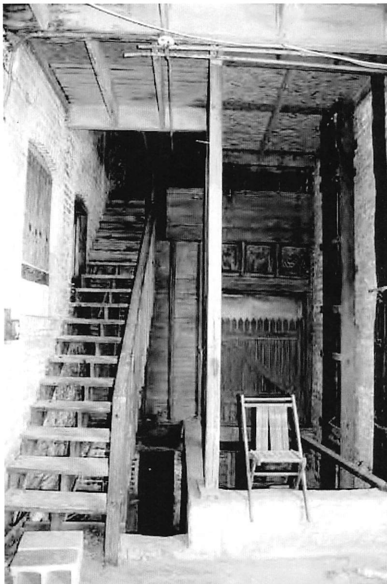
9 of 28: Interior view of nonhistoric rear stair and historic casket elevator; photographer facing northwest.
